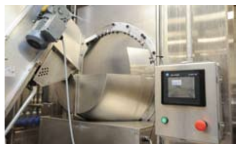
An Allen-Bradley PanelView 600 control panel and SEW-Eurodrive motor help power a cap distribution system on Gay Lea’s aerosol packaging line.
